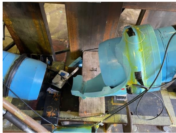
(c) Failure on fitting
