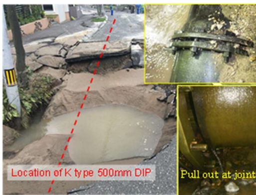
Photo 5. Damage to 500 mm-diameter pipe.
