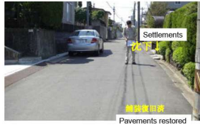
Ground surface of damaged pipe location (D100DIP, leakage from joints: Nankodai, Sendai, Miyagi pref.)
