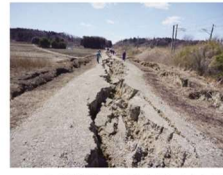
Fig. 34 パイプ敷設道路の亀裂 (矢吹南第2空気弁工周辺) Cracks on the road around Yabukimami No.2 air valve
