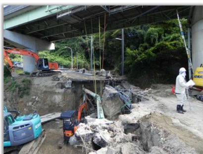
Photo 3. Mudslide site in Yano
