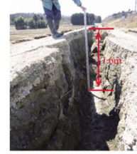
Fig. 35 パイプ敷設道路の亀裂 (矢吹南第2空気弁工) Cracks on the road around Yabukimami No.2 air valve
