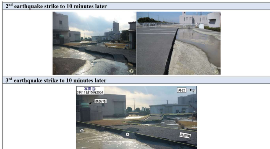
Figure 10. Time sequence of damage at Wanigawa WTP, Ibaraki Pref. after the main shock of the 2011 Tohoku earthquake (Iwatsubo et al. 2023).
