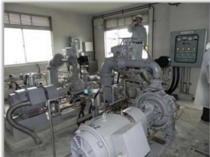
Photo 1. Maki purification plant
