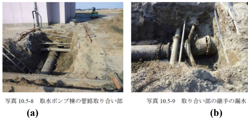
Figure 11. Complex pipeline damage at Wanigawa WTP, Ibaraki Pref. after the main shock of the 2011 Tohoku earthquake (Kuwata and Katagiri, 2022)
