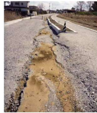
Fig. 45 パイプ埋戻し材料の噴砂 (矢吹北第5排泥工周辺) Sand boil on a road around Yabukikita No.5 blow off
