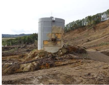
Figure 12. Damaged water storage tank at Tomisato WTP, Atsuma-town, Hokkaido after the 2018 Hokkaido Iburi-Tobu earthquake.
