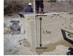
Fig. 36 矢吹南第2空気弁工の浮上 Uplift of Yabukimami No.2 air valve
